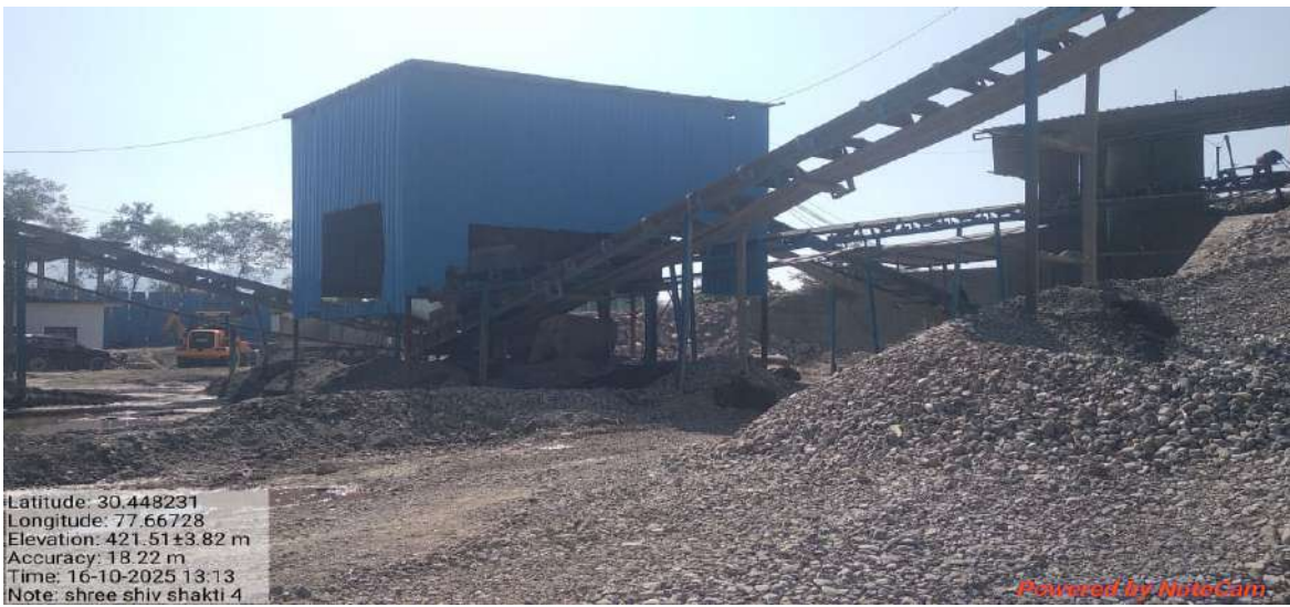
All conveyor belts not covered.
