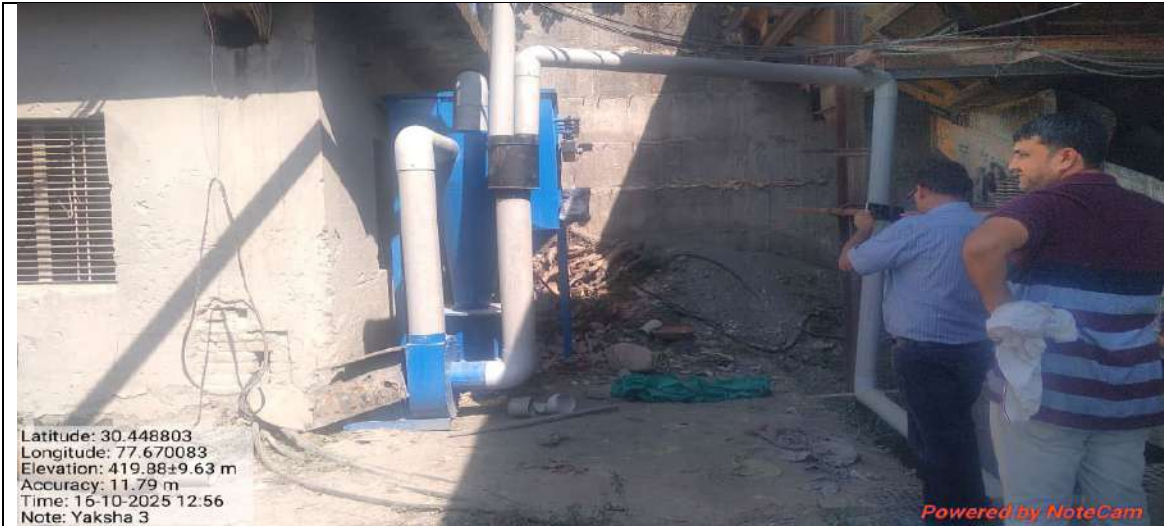
Bag filter and cyclone
