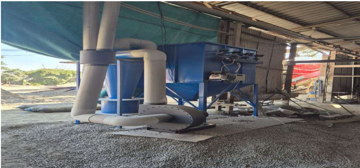
Bag filter and cyclone
