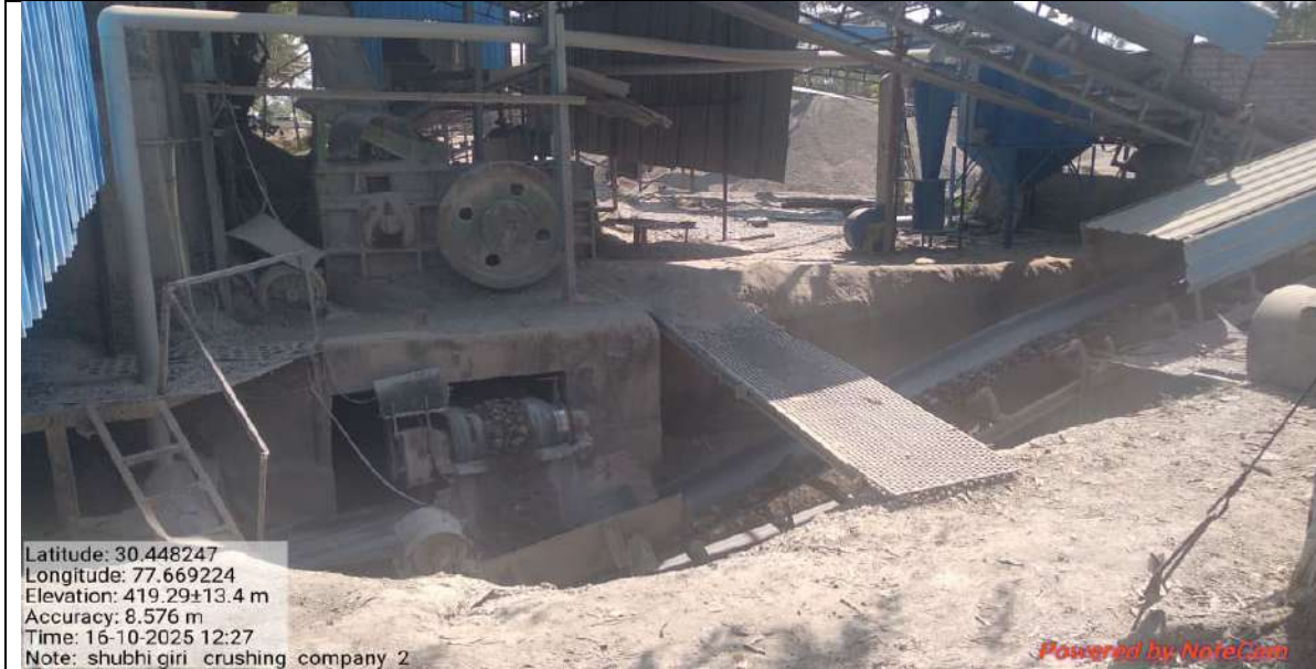
Bag filter and cyclone
