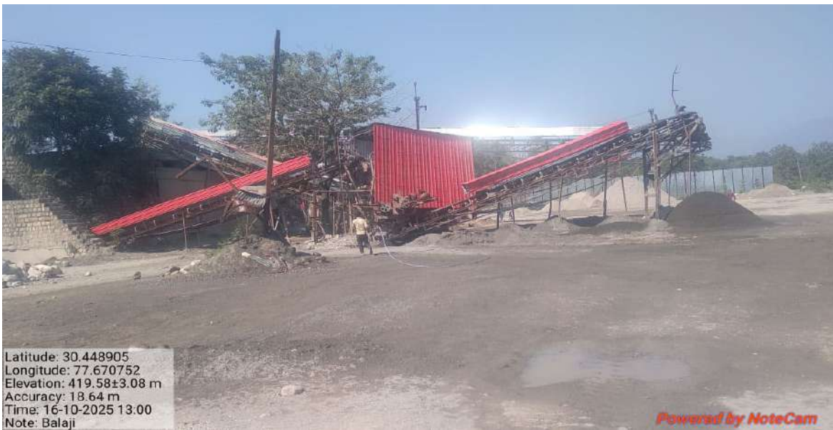
Conveyor Belts for wet material transfer
