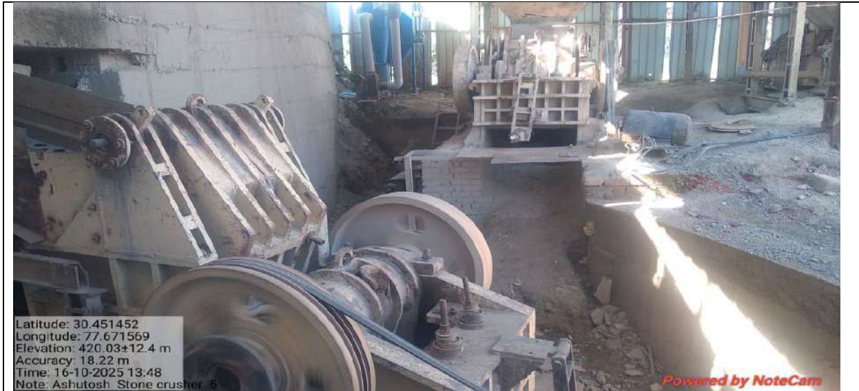
Primary and Secondary crusher partially covered.
